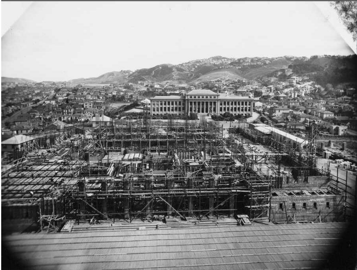
Photograph 9.3: Dominion Museum, Wellington, under construction. Smith, Sydney Charles, 1888-1972: Photographs of New Zealand. Ref: 1/1-023103-G. Alexander Turnbull Library, Wellington, New Zealand. /records/22704214
