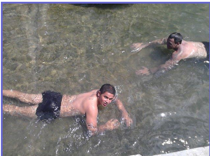
Pte Morris-Kerie and a Naval Leading rating doing a Underwater check of the Slipway for integrity.
